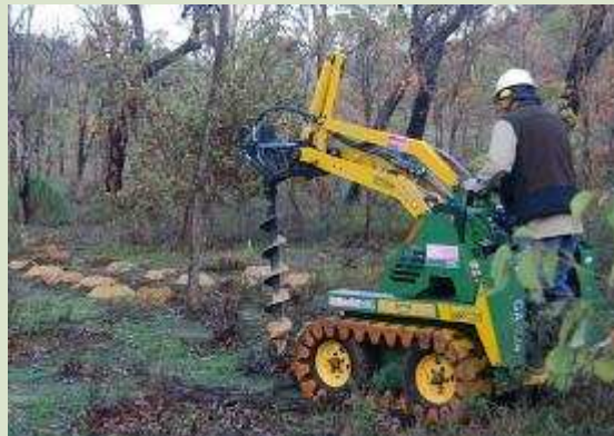
Post-hole digger in action at Helena River in June 2011. Photo – Penny Hussey
